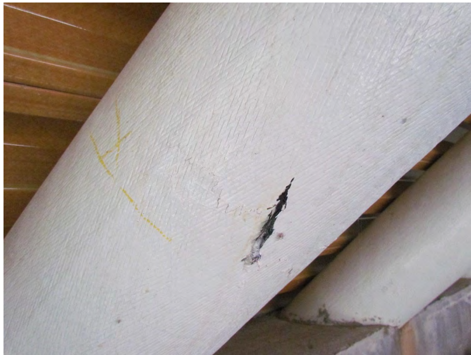
Figure 23: Example of Laminate Penetration
